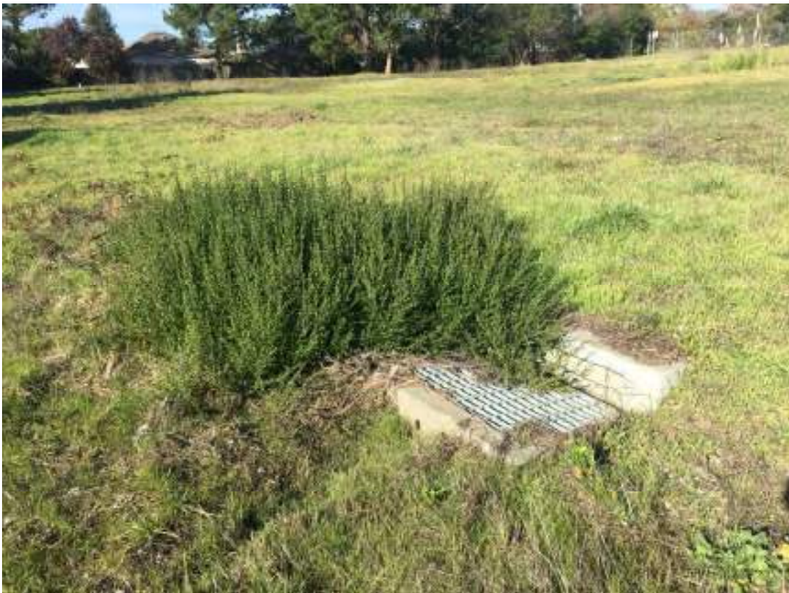
STORM SEWER INLET AJDACENT TO SOUTHERN BORDER OF PROPERTY
